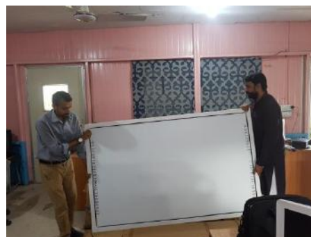
Figure 16 e-learning installation in Darkala
